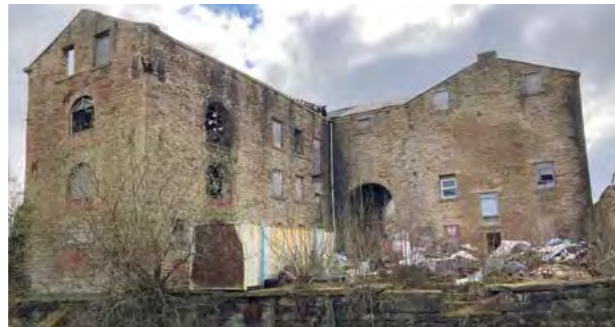
Hargreaves Warehouse, Grade II listed building in a state of dereliction, Church & Oswaldtwistle
